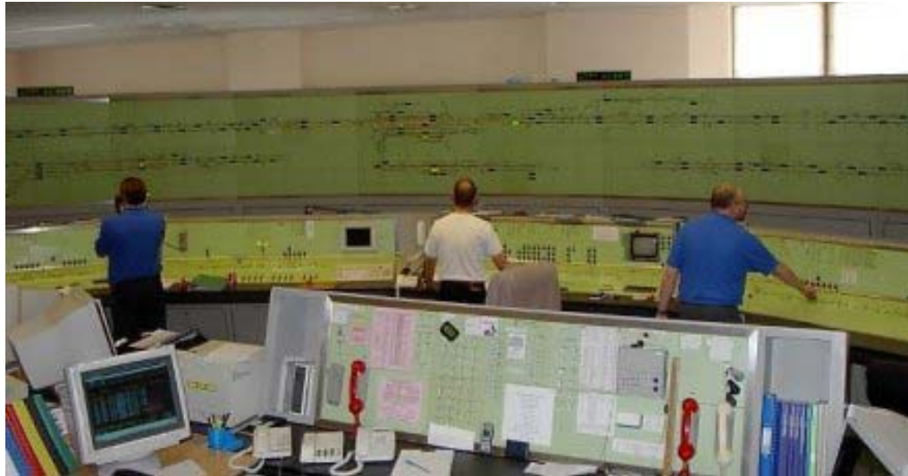
• Photo 2.2 Large Power Signal Box at Exeter, © P.S.Bellamy
